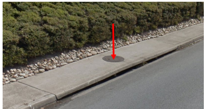
SCDOT Type 18 Catch Basin
