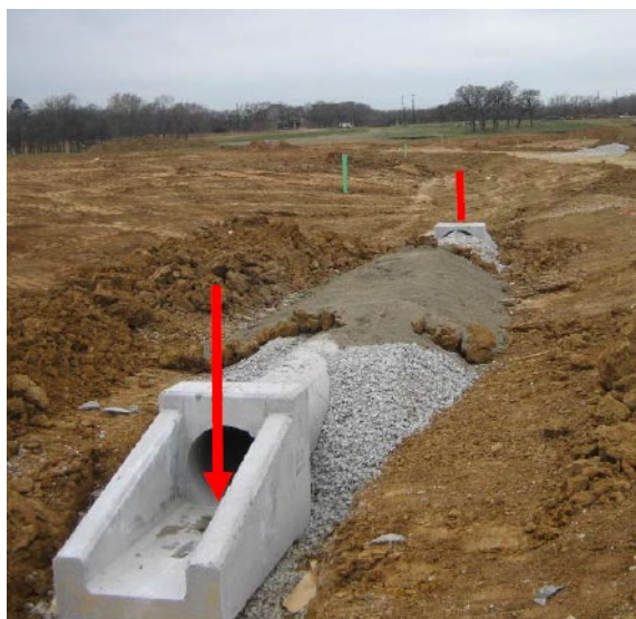
Figure 64 Example Storm Sewer Pipe
