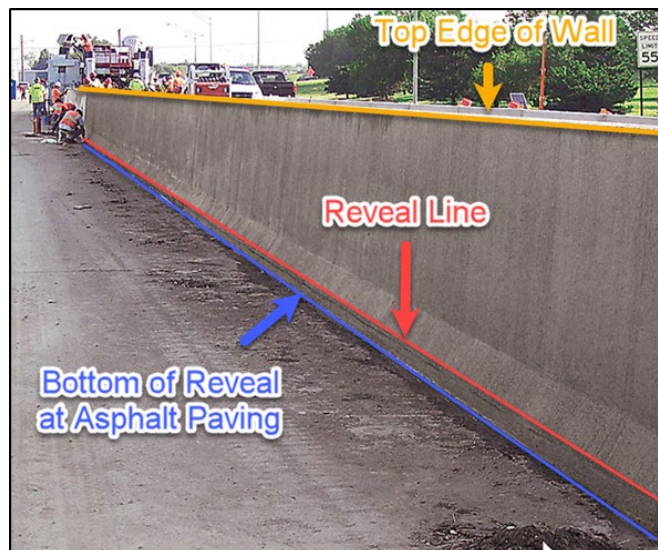
Figure 10 Interstate 3D Breakline along Reveal Line, Bottom of Reveal at Asphalt Paving, and Top of Wall
