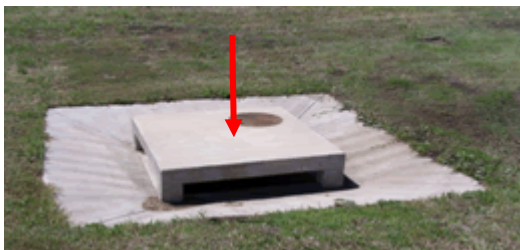
SCDOT Type 9 Catch Basin
