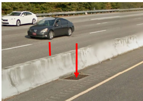
SCDOT Type 15 Catch Basin
