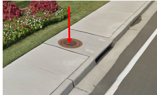
SCDOT Type 16 Catch Basin
