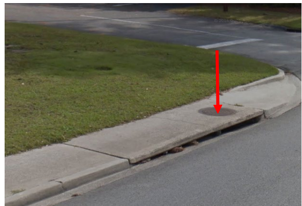
SCDOT Type 17 Catch Basin
